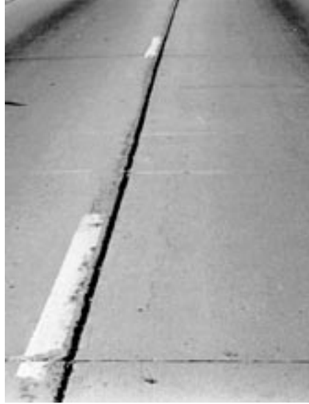
▲ Joint open about 1/2".
