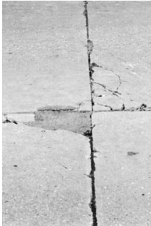
▶ Broken corner pieces. Some joint spalling.
