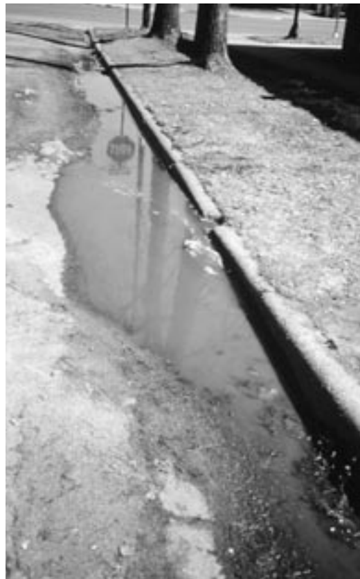
► Flooding. Curb and gutter need reconstruction.
