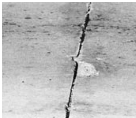
◀ Moderate spalling at transverse joint.
