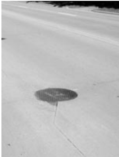
▶ Isolated spall at manhole.
