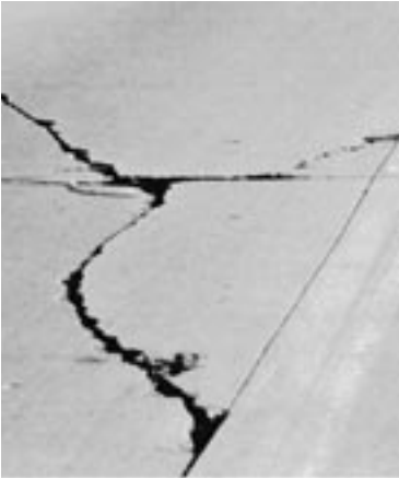
Wide open meander crack (1") with edge spalling. ▼ Corner crack with spalling.
