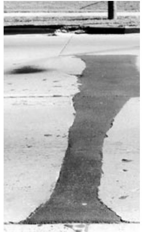
Patching in ▼ fair condition.
