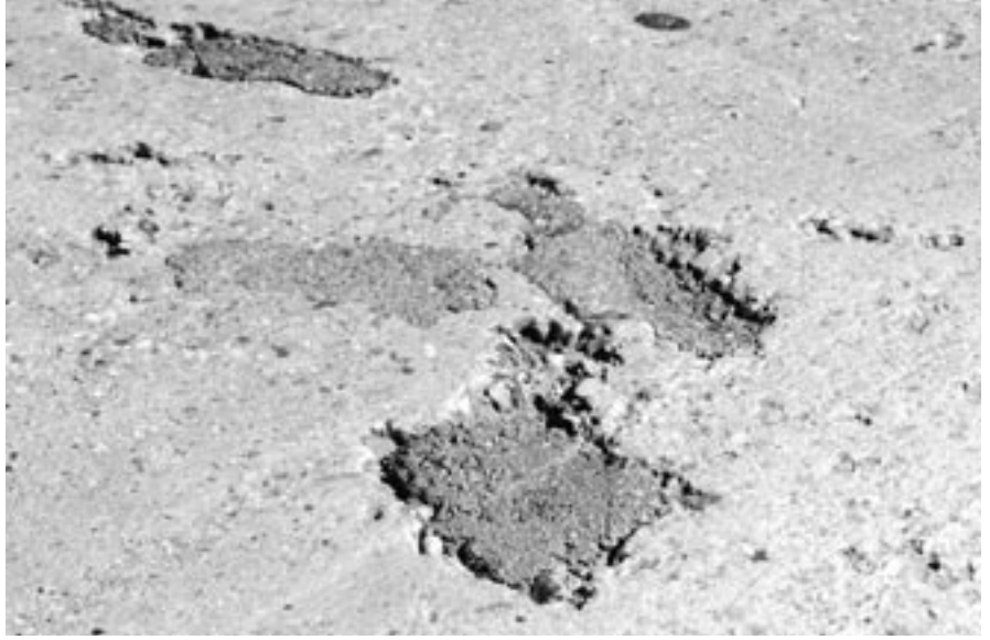
▶ Small surface spalls that have been patched.
