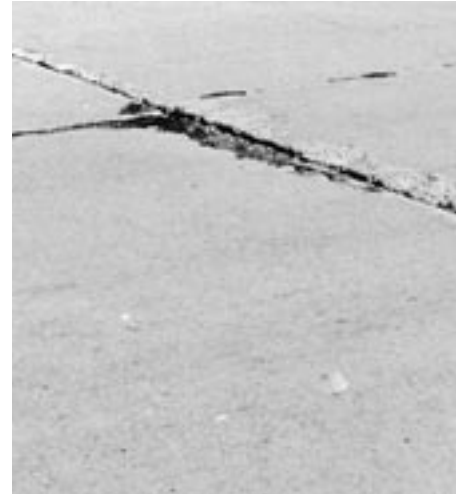
▼ Transverse joint has slight faulting and spalling.
