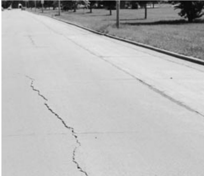
► Settlement caused meander crack with faulting.
