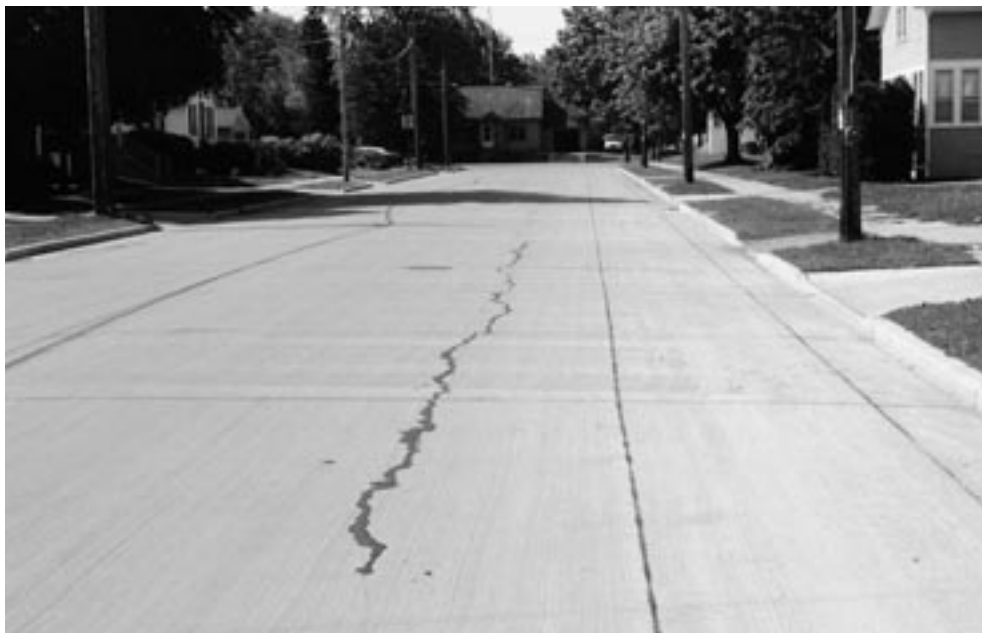
▶ Isolated meander crack, tight and well sealed.
