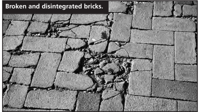
Open joints and broken brick at utility cover.
